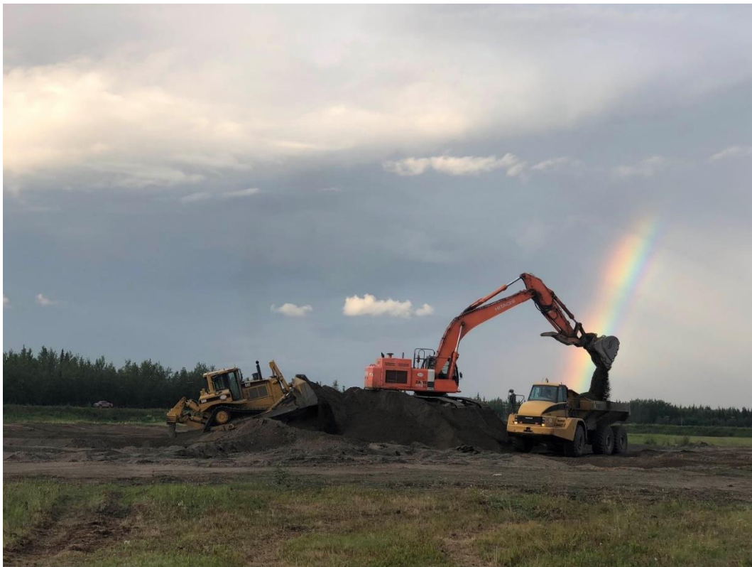
Galena Airport excavation at the end of the rainbow, August 2018 Photo by: Larissa Figley
