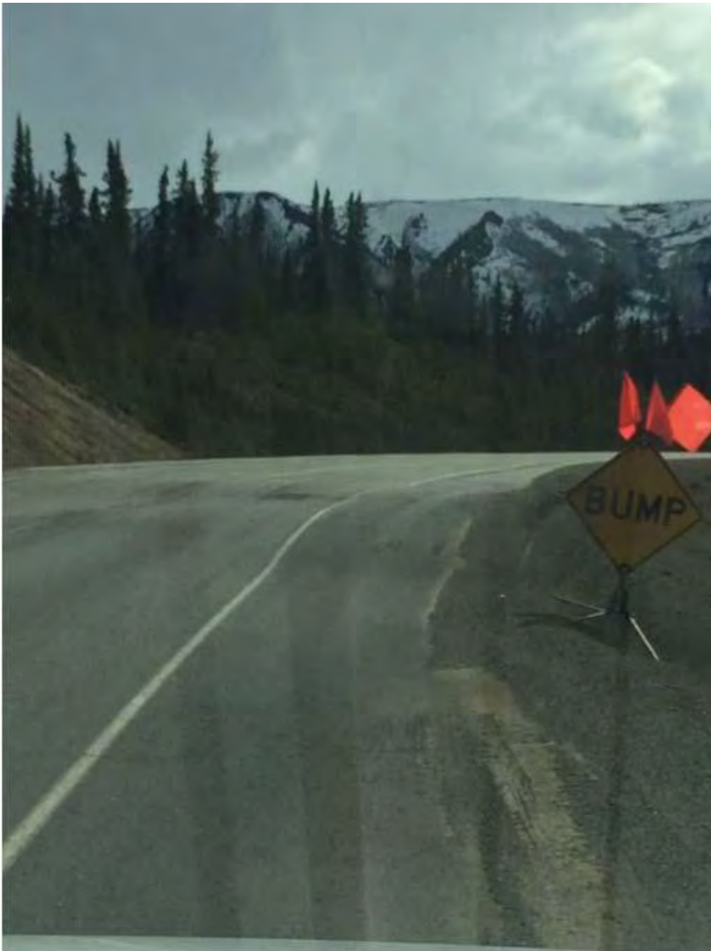
Roadway settlement [near MP 232.5]
