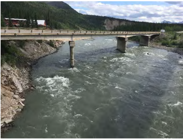
Nenana River Bridge between Glitter Gulch and Denali Park entrance turnoff - some erosion of the left riverbank visible
