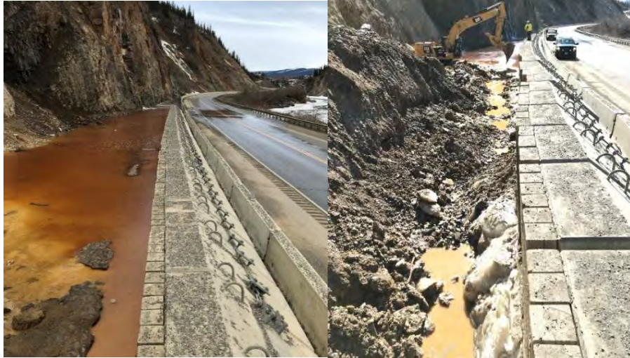
Figure 48. Drainage issues from slide debris behind concrete barriers
