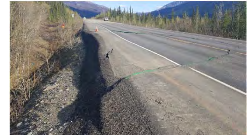
Extreme thaw settlement (~MP 235)
