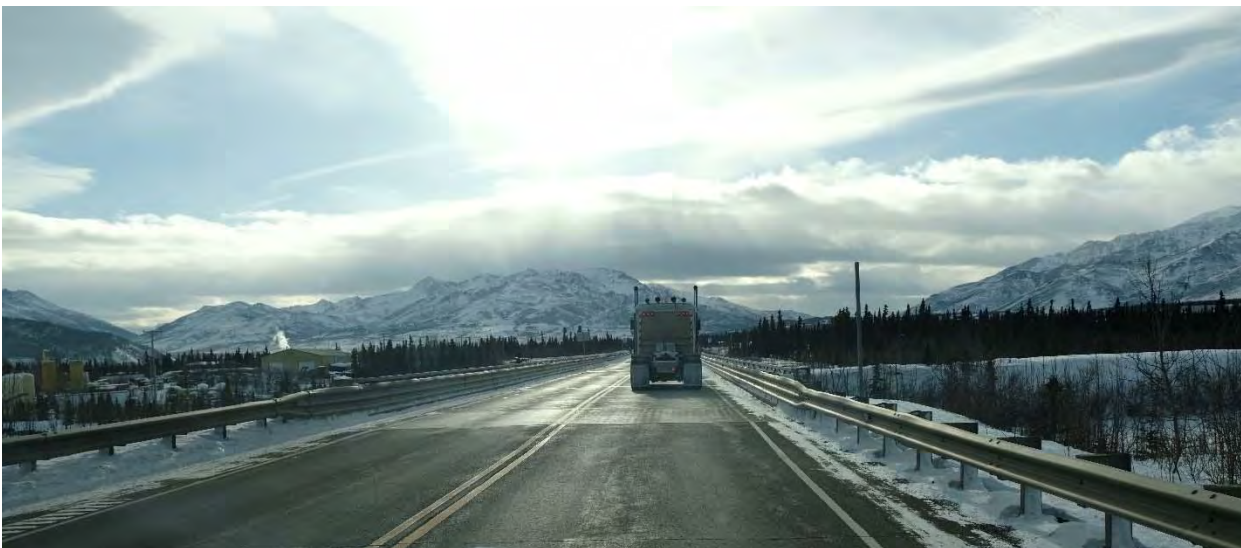
Dry Creek bridge has narrow shoulders (near MP 250)
