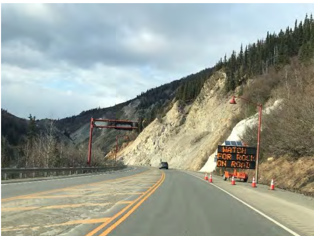
Nenana Canyon rockfall hazards (MP 239-241)
