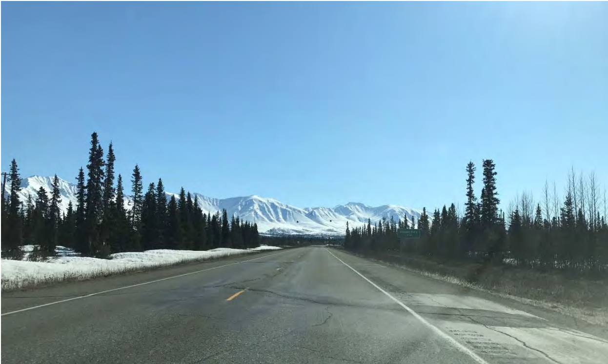
Roadway condition: pavement cracks (MP 211)
