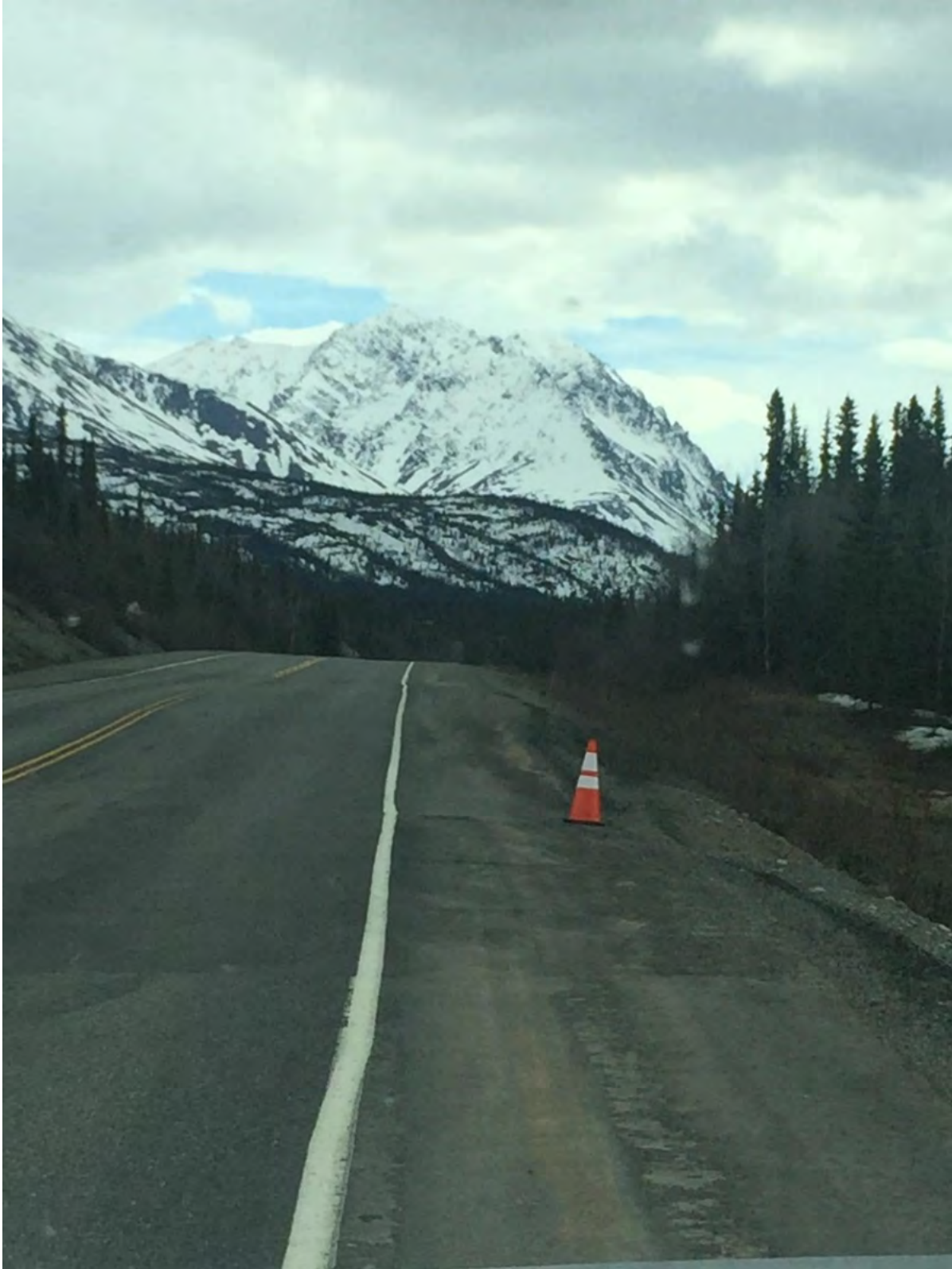
Figure 5 – Section near MP 228.5, where the road is settling
