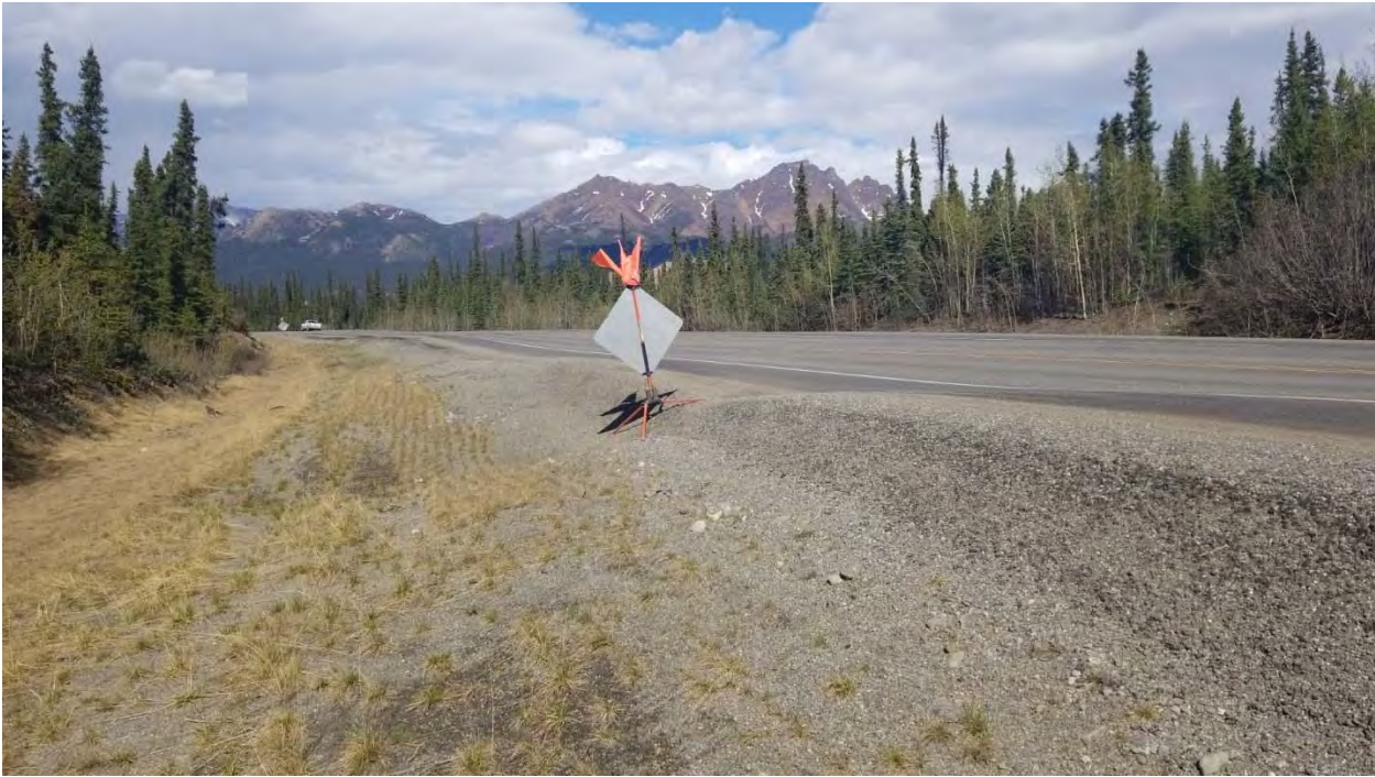
Example of roadway settlement (MP 233.5)
