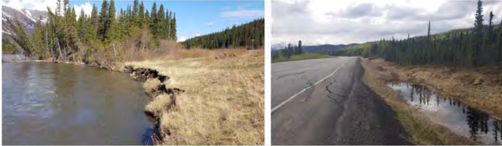
Bank erosion from Nenana River adjacent to the Highway (MP 222.8) (Left), Roadway deterioration adjacent to thaw pond, likely caused by thawing permafrost (MP 256.4) (Right)
