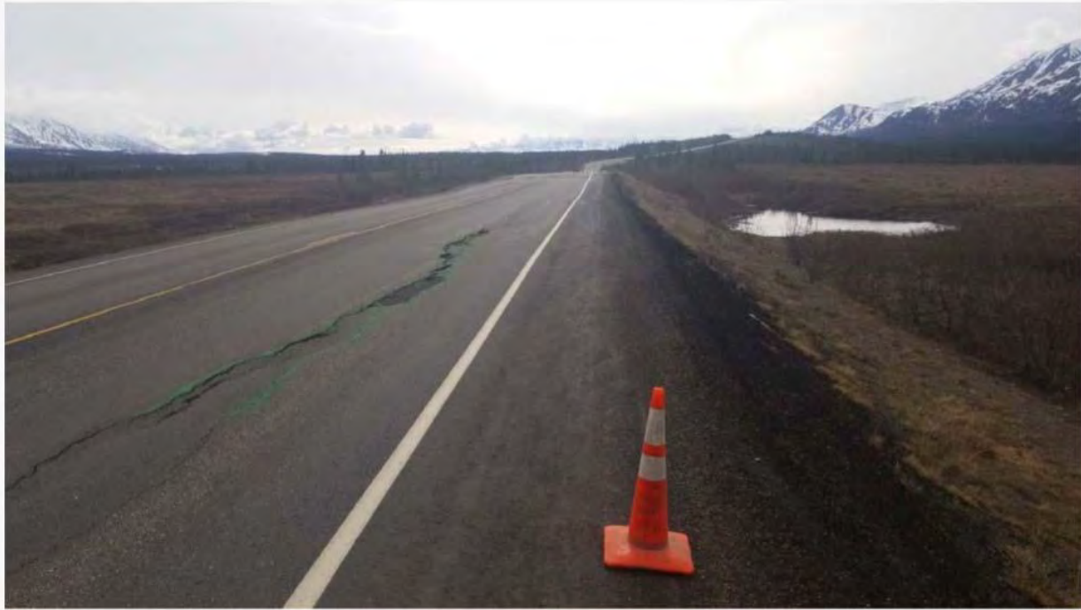
Example of pavement damage and frost heaves near MP 206
