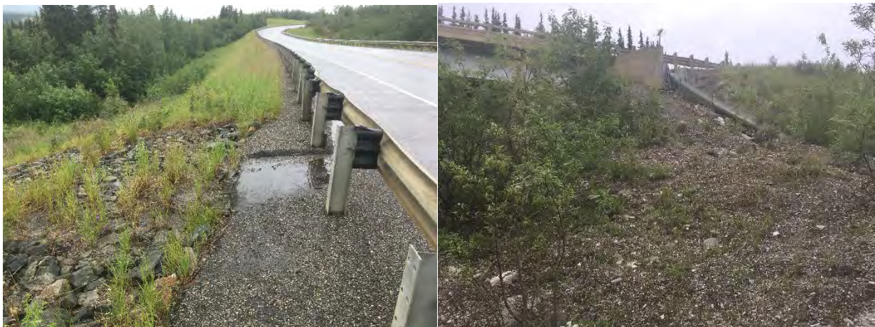
Figure 62. Typical Riprap Flume Looking Toward Slate Creek: Typical Metal Flume on Southbound Side of the Kingfisher Creek Crossing
