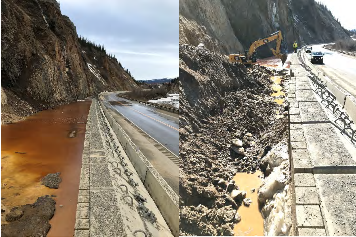
Figure 18 – Drainage issues from slide debris behind the jersey barriers
