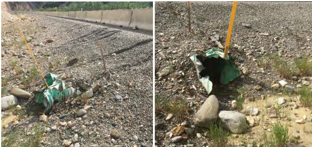
Figure 49. Damaged Culvert End Condition near MP 239.5 on the East Side
