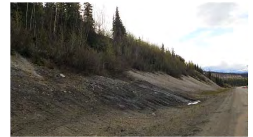
Unstable cut slopes (~MP 238)
