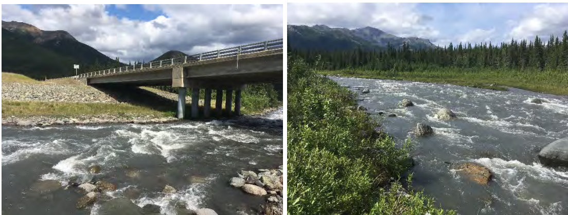
Figure 15. Riley Creek Looking Downstream, At Left Abutment, Looking Upstream from Left Abutment
