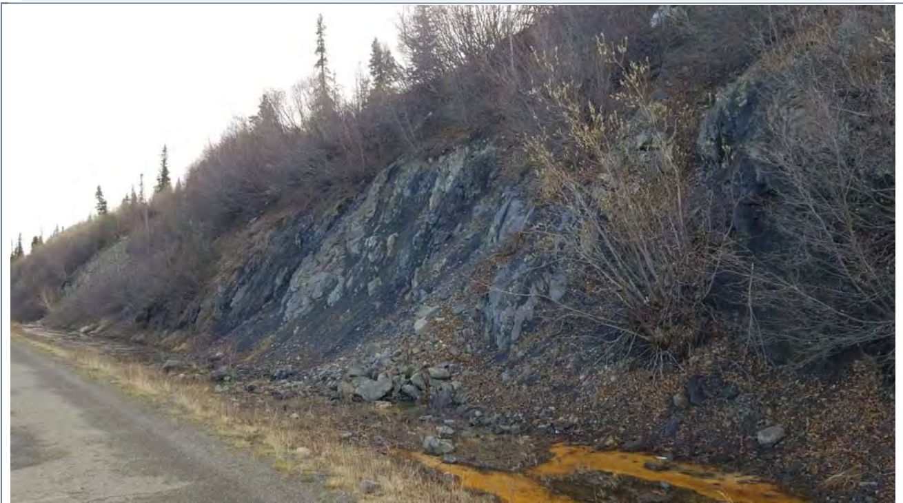
Photo 6: MP 212 Unstable soil and rock slope. Vern Carlson (Maintenance Foreman) stated that the site was a slow-moving slide that caused the ditch to be cleaned out every three to five years depending on rainfall.
