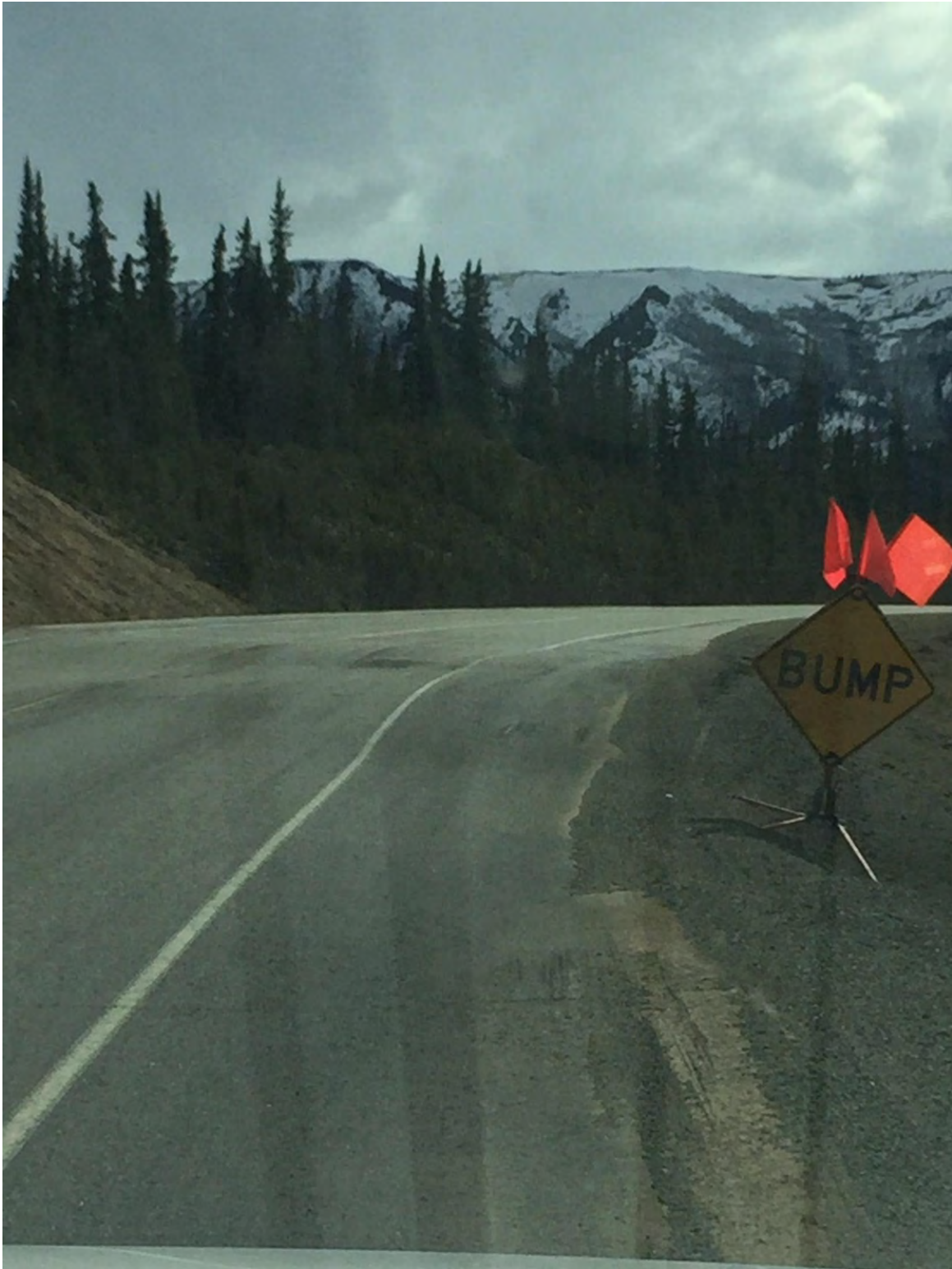
Figure 6 – Annually reoccurring bumps around MP 232.5, likely caused by an ice lens
