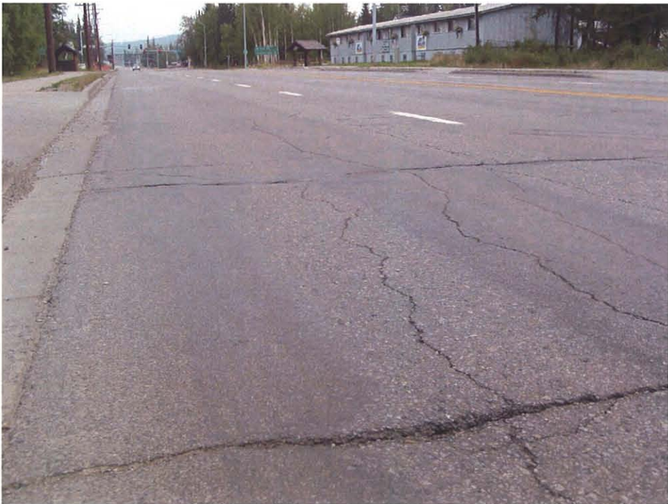
Figure 1.2.4.3 Pavement Cracks –University Avenue
