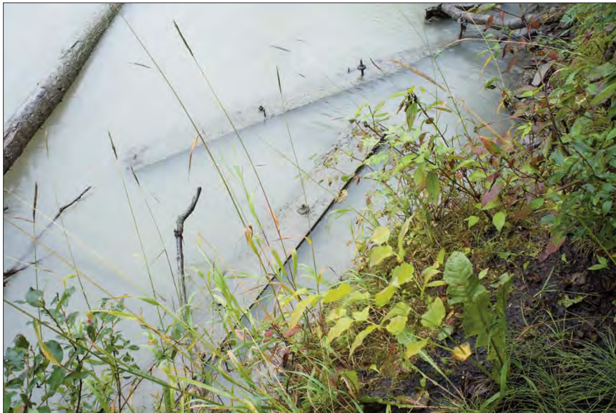
Figure H-7. Sway braces in the the Chilkat River at the location of the first Wells trestle.
