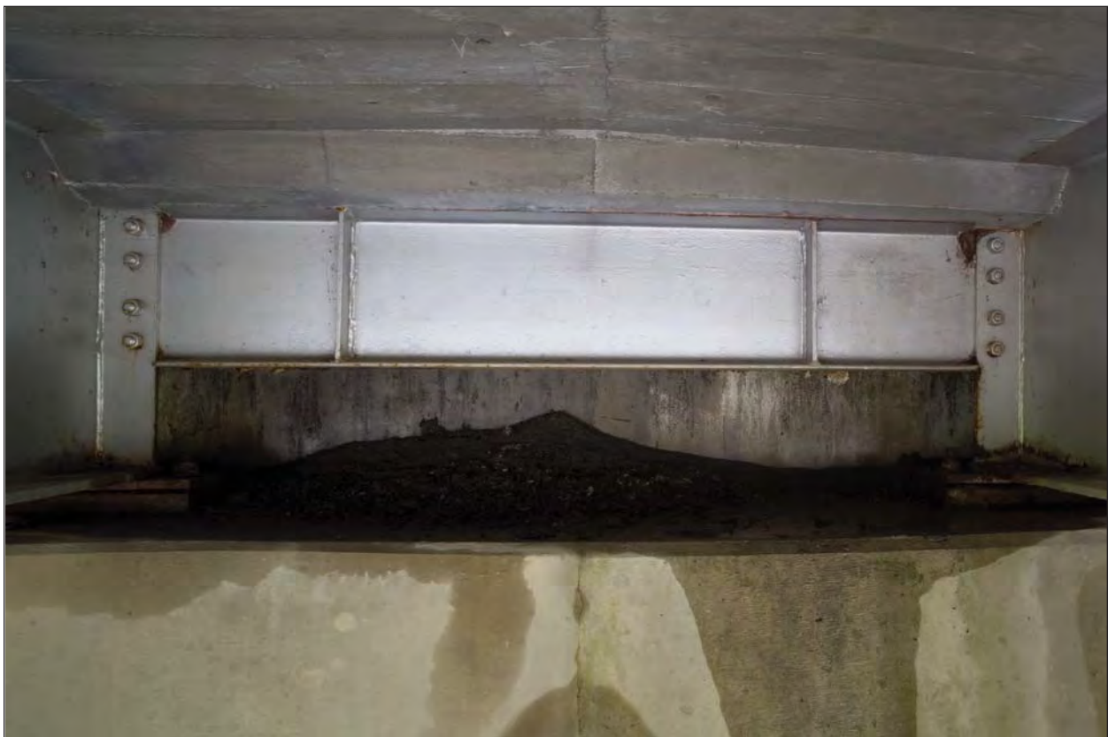
Figure H-13. Peaked roadway crown and north abutment.
