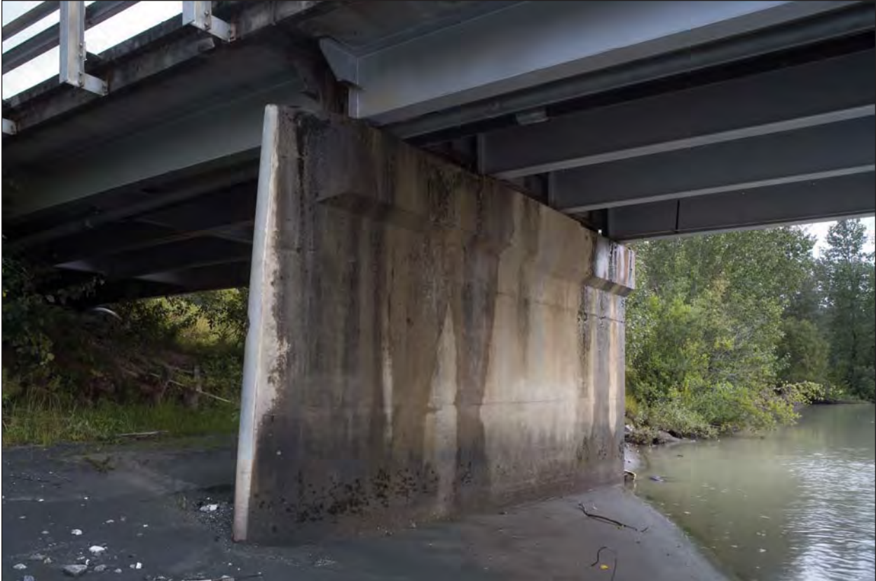
Figure H-14. Upstream end of one of the concrete piers with a steel face showing the short channel sections welded to the stringers to support the curb.
