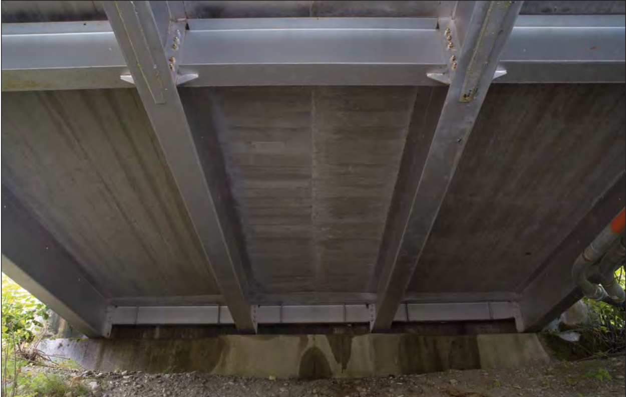
Figure H-16. Form marks on the underside of the concrete roadway showing the sequence of the concrete deck pour.
