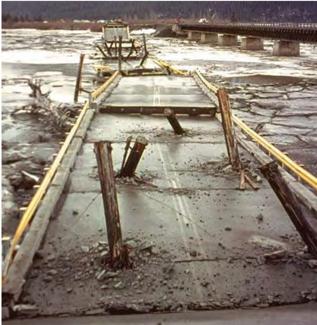
Figure 5 - Earthquake induced bridge damage (Alaska 1964)
