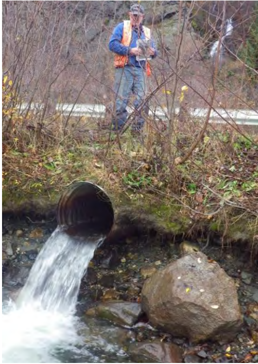
Figure 2. Bob Trousil stands above perched culvert. Waterfall in the background (October 25, 2013).
