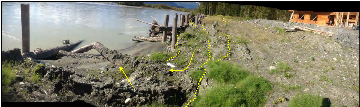
Figure 6. Wood/soil revetment structure along the Chilkat River, Klukwan, Alaska. Dashed lines indicate approximate locations of longitudinal cracking of the ground surface in the immediate area. Arrows indicate direction of bank slumping and material loss. (ADOT&PF August, 2013).
