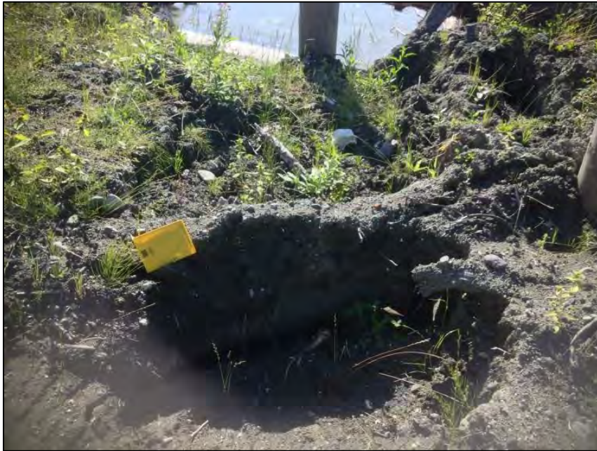
Figure 7. Void formation and slumping at upstream end of wood revetment, Klukwan, Alaska, (ADOT&PF, August 2013).
