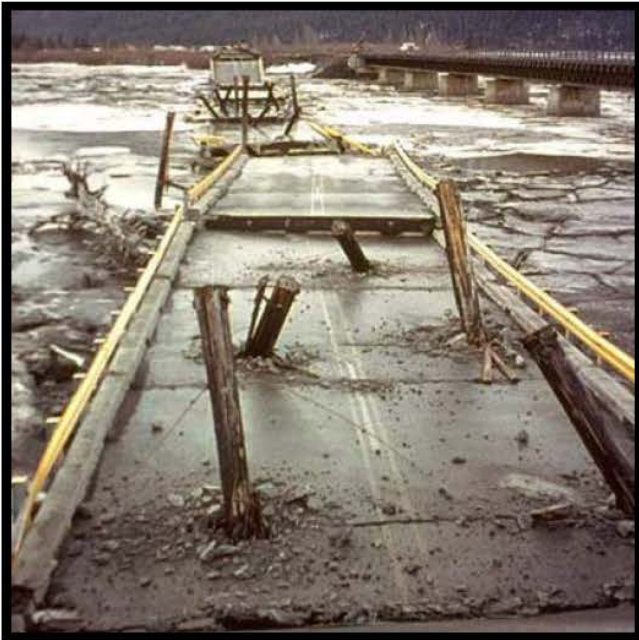
Photograph 2: Example of Bridge Damage from Earthquake
