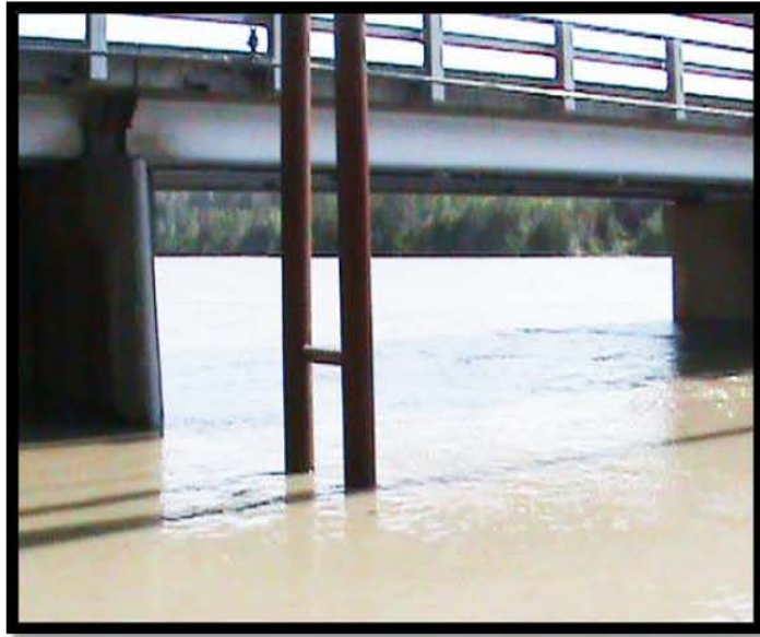
Photograph 3: Bridge Low Clearance
