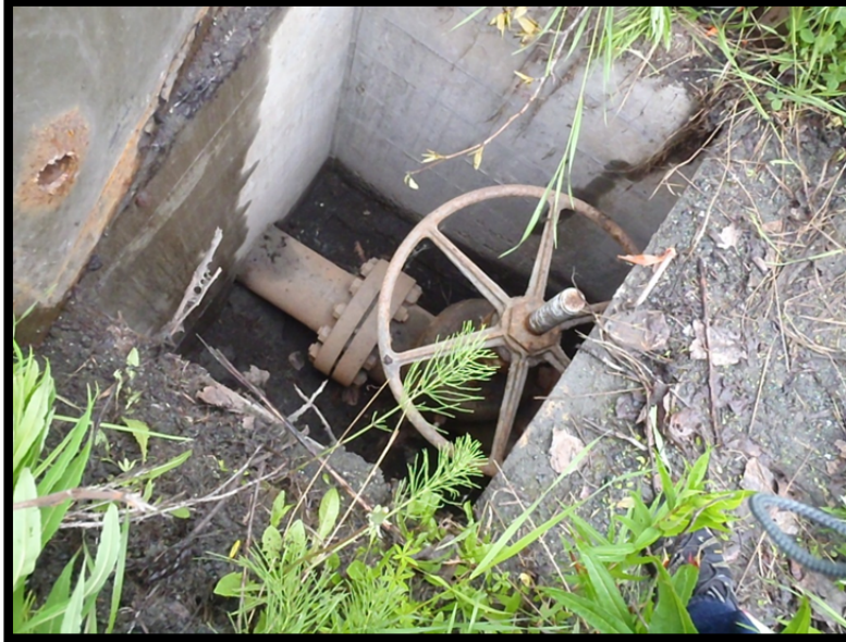
Photograph 4.10-1: Haines-Fairbanks Pipeline Gate Valve 4
