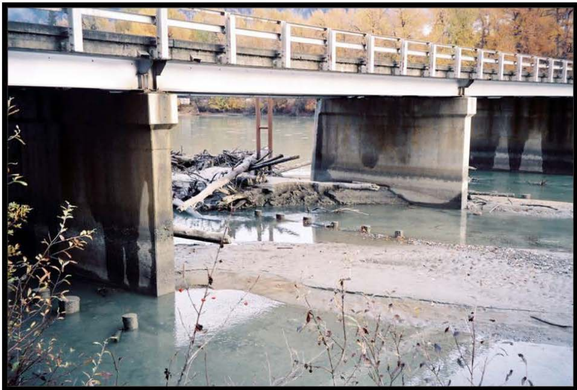
Photograph 4: Logjam Underneath Bridge
