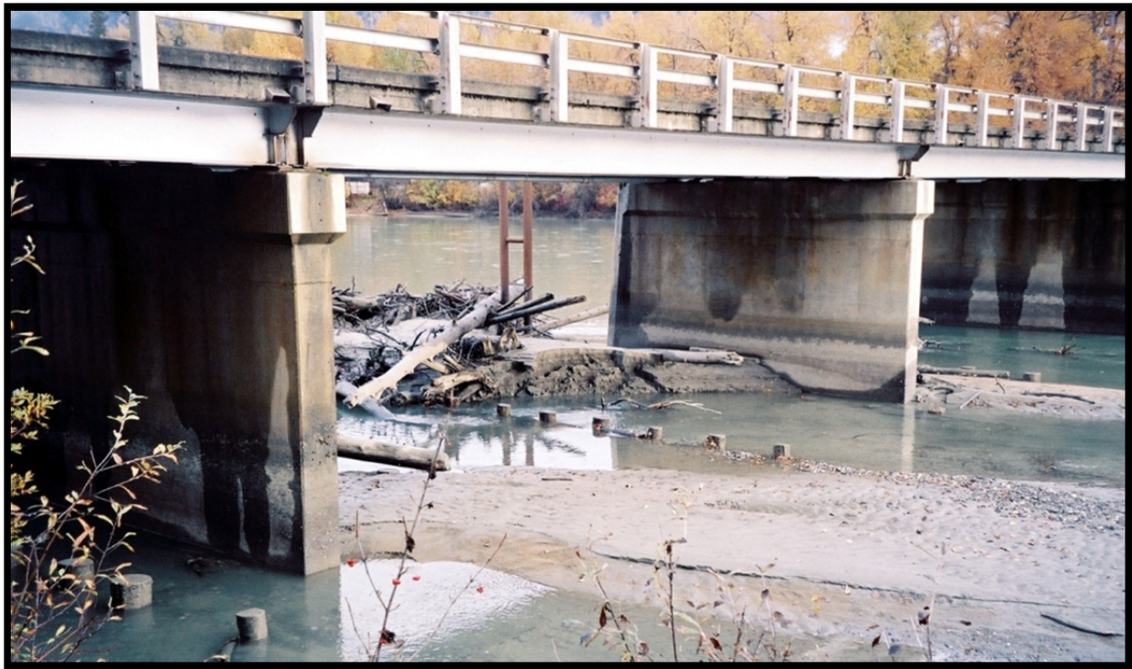
Photograph 4.12-1: Logjam Underneath Bridge
