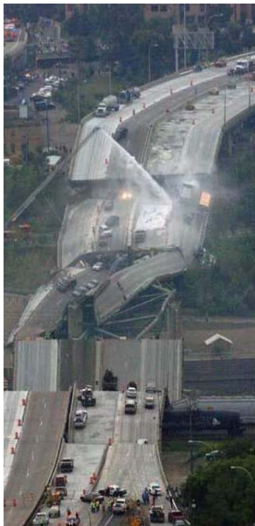
Exhibit 35. I-35W bridge collapse in Minnesota
