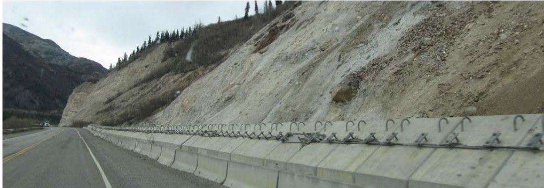
Exhibit 24. Rockfall protection system
