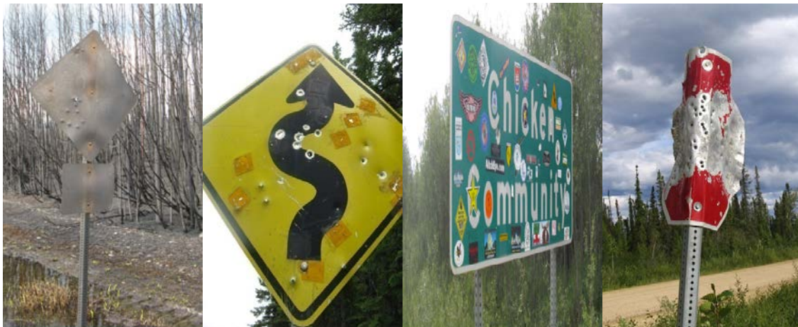
Exhibit 33 Examples of unacceptable signs (Alaska DOT&PF 2011)
