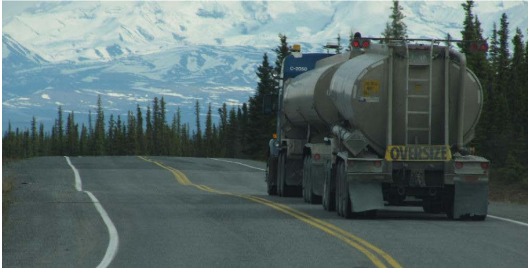
Exhibit 48. Long-wave unevenness caused by permafrost and freeze/thaw
