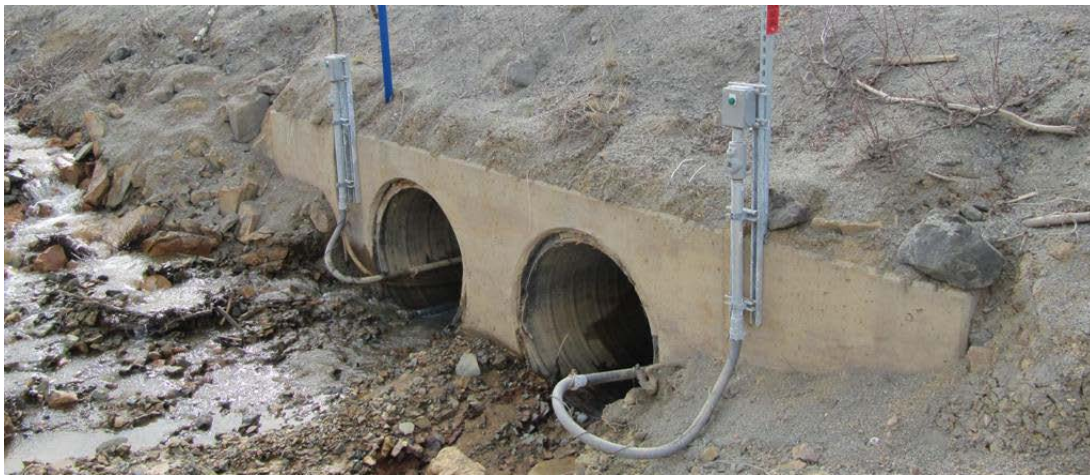
Exhibit 25. Culverts with heating systems
